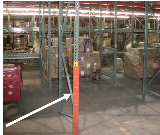
Damaged column with home-grown repair
