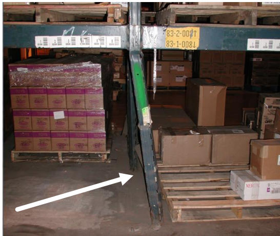
Damaged upright column
