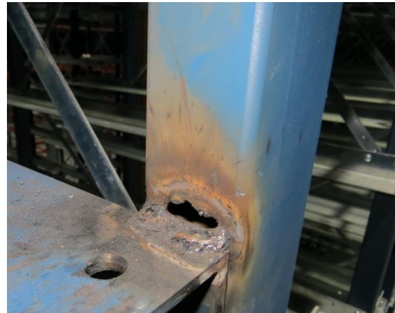
Defective field welding
