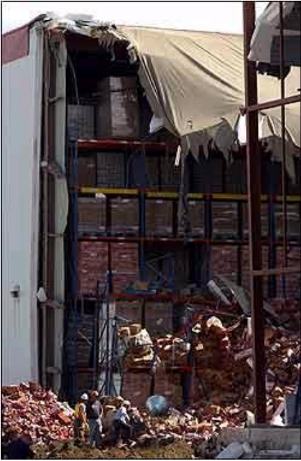
Rack collapse led to the surrounding building's collapse
