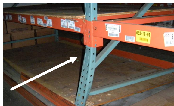
Damaged upright column
