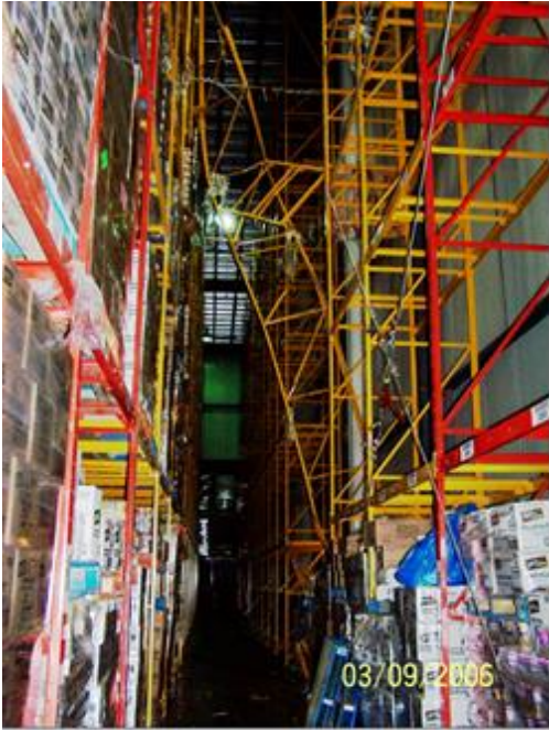
Rack damage was ignored
