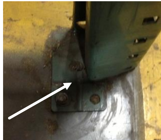
Sheared anchor; footplate separated from column
