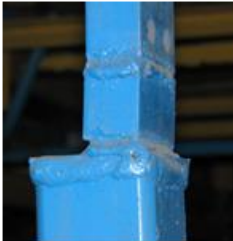
Unsafe field welding repair
